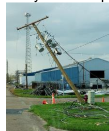
Power system damage in Town of Iowa, Louisiana
